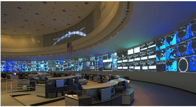
Fig. 10. Display Wall of the AT&T Network Operations Center.
